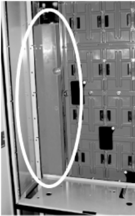
Bus Splice Access Cover In Place
