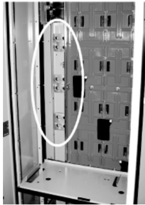
Bus Splice Access Cover Removed
